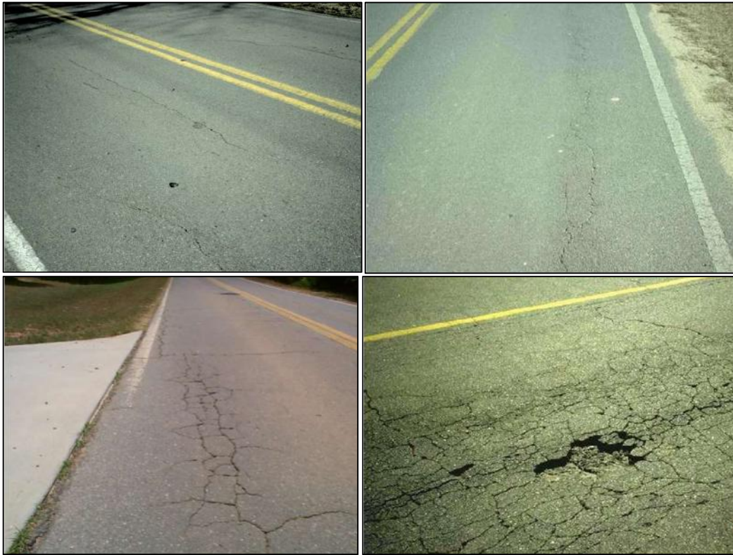
Figure 1: Crack Severity levels for load cracking. Level 1 (top left) to Level 4 (bottom right)
